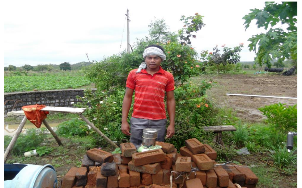
Installation of rain gauge
